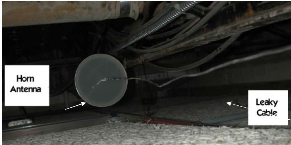
Figure 5: Leaky Cable Installation in Crowded Ceiling Space
